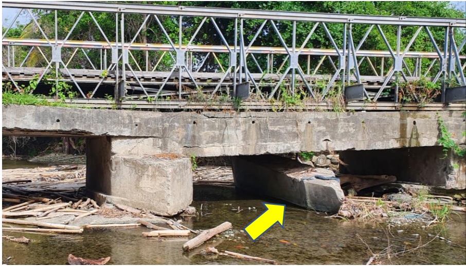
(a) Seamoon Bridge (SB on Fig. 1(a)): Tilted Support
