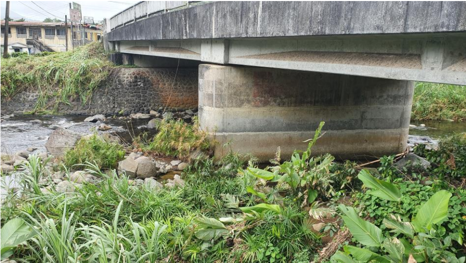
(b) Birch Grove Bridge (BirB on Fig. 1(a)) : Mid-River Support and River Wall Work Well
